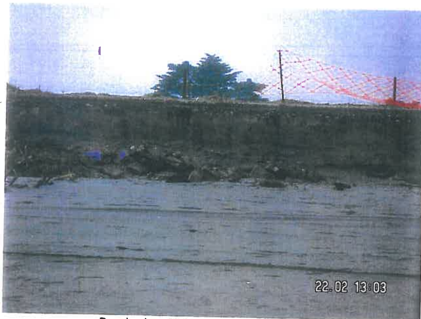
Road edge, limited rock toe protection
