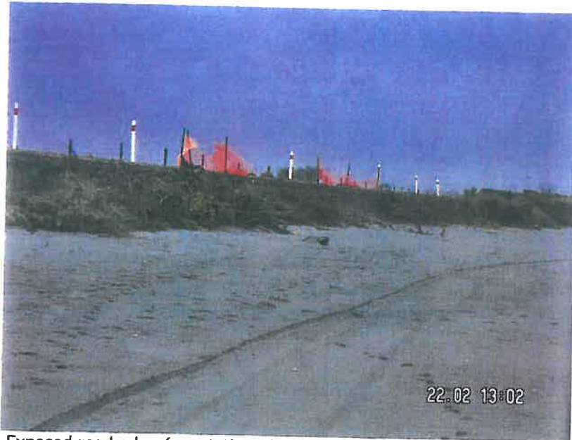
Exposed road edge (vegetation placed in attempt to protect the bank)
