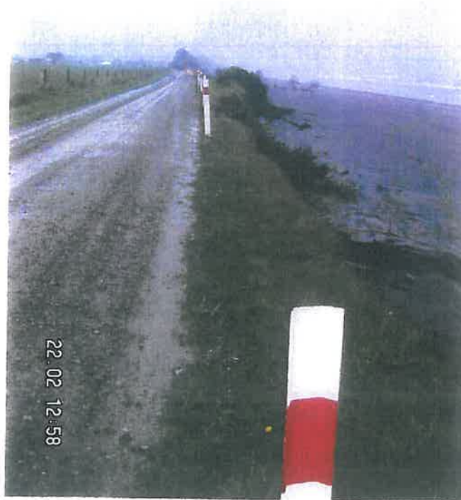
Erosion scarp relative to Rotary Drive
